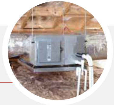
Indoor Fan Coil Unit installed within a roof space
