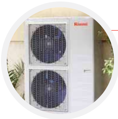
Outdoor Condensing Unit
